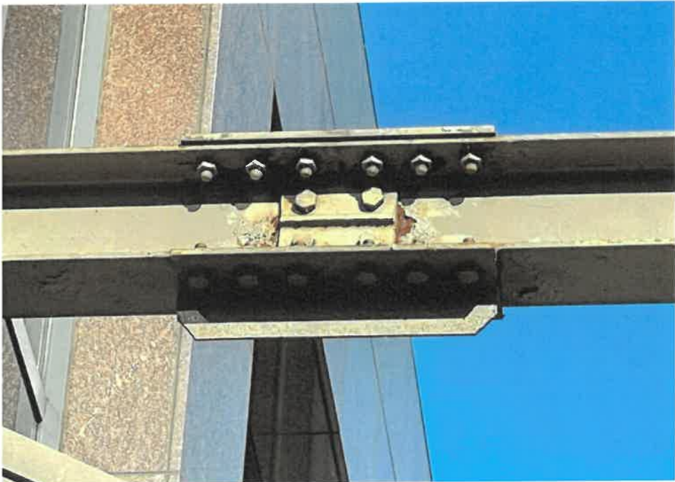
Photo 12: - Corrosion of steel in web of beam at moment splice connection.
