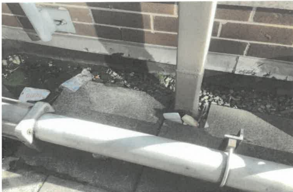
Photo 10: - Algae growing around the base of the HSS 4x4 post columns.
