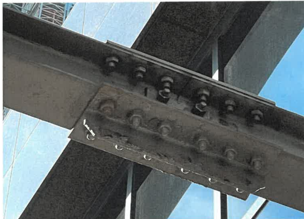
Photo 8: - Peeling paint & surface corrosion on underside of beam moment splice located at catwalk level.
