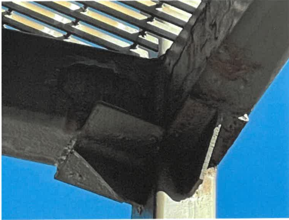
Photo 9: - Surface corrosion on the underside of north most beam and supporting bracket for the catwalk level framing.
